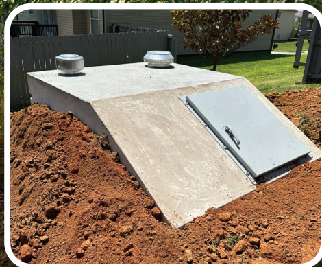
Concrete Tornado Shelter 6' wide X 8' long X 6'2" tall
