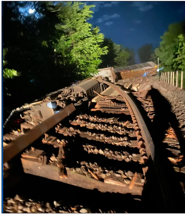
fallen onto the tracks. The collision caused 31 railcars to derail in various positions, including two locomotives.
